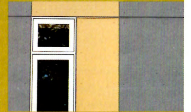
The fiber cement panels were installed wrong-side out and painted gray.
